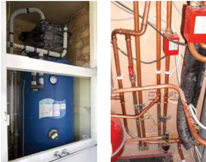
Figure 8. Two solar water heating systems showing good (left) and poor (right) levels of insulation
